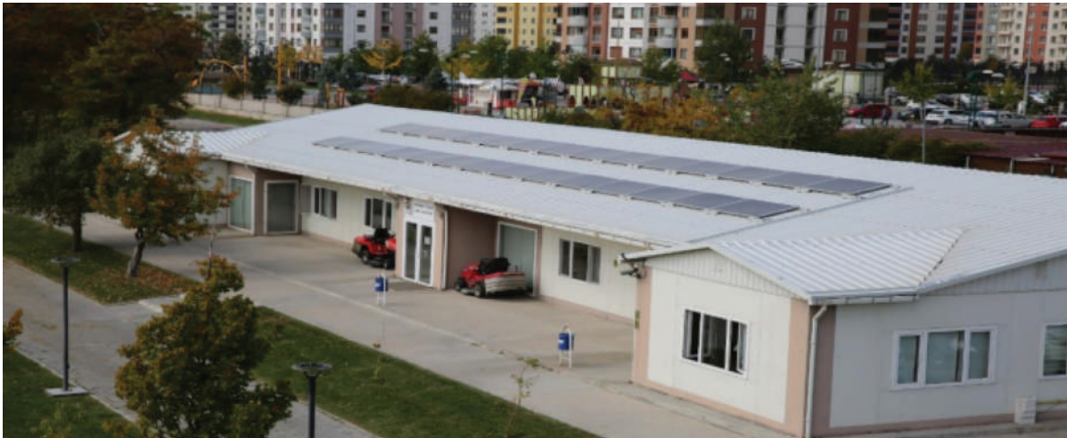
The Solar Power Plant Built on the Department Building's Roof
